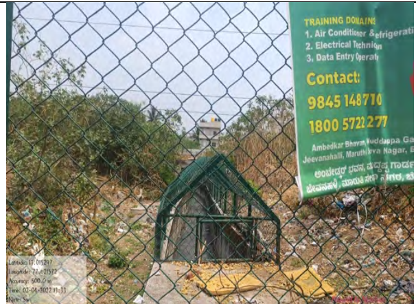
SW10 Drain near Whitefield
